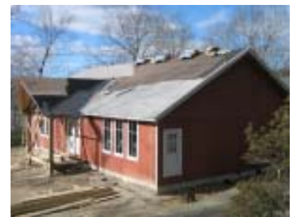
The new addition is taking shape now and the Capital campaign is in full swing. The building will be dedicated on April 29, 2006
